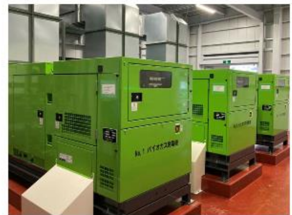
Generators that generate electricity using methane gas
