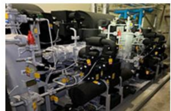
Karatsu Logistics Center's non-CFC freezers
