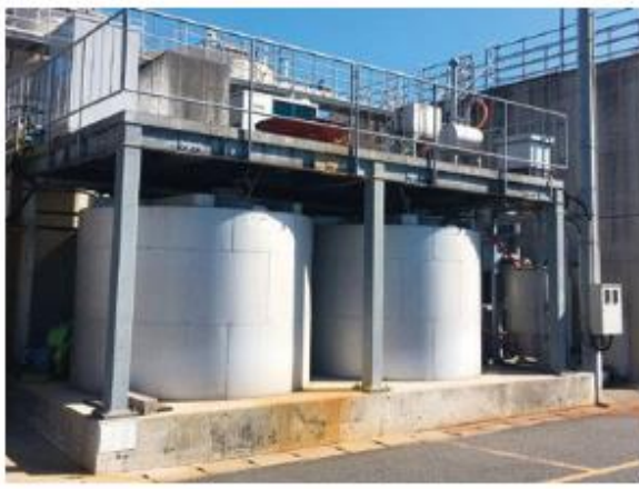
Shimonoseki plant biogas power generator
