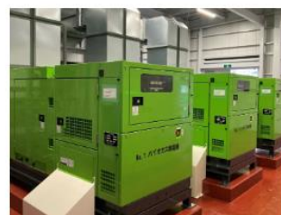
Generators that generate electricity using methane gas
