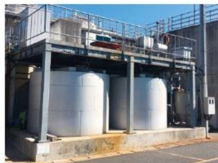
Shimonoseki Plant biogas power generator
