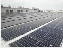
(Reference) On-site solar panels installed in 2021 at Utsunomiya Plant
